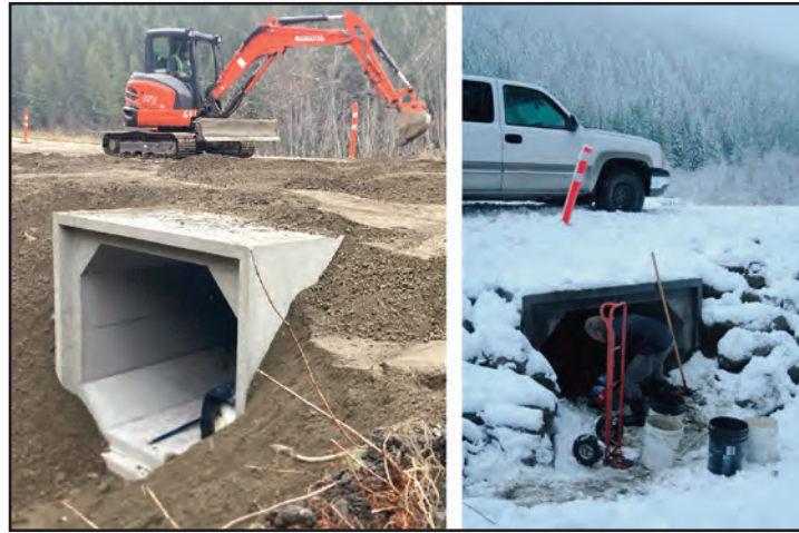
Left: New box culverts being installed under Highway 31A that will help reduce traffic mortality to Western toads and many other species. Black bears will also be able to use them. Right: Worker installing sand for the floor of the cement culvert.
